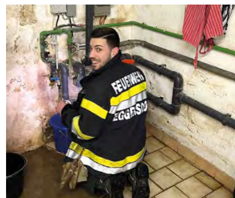
Wasserrohrbruch in Eggersdorf
